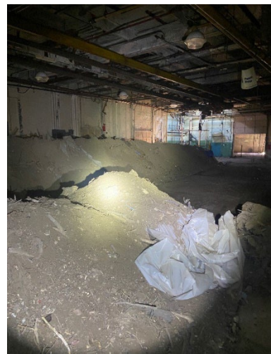
Figure 2. Soil stockpile located within the building. Photo: Sean O'Donnell, August 2024
